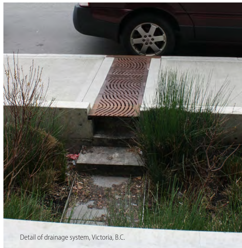
Stormwater management system between two Pedestrian Through Zones in Victoria, B.C.
